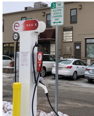
New EV charger at Main and Wing parking lot. Photo by Lori Ward.
